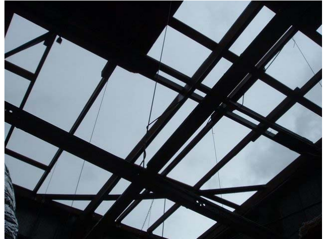
DESTROYED CEILING & ROOF
