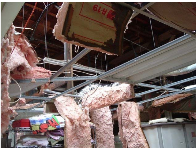
COLLAPSED CEILING & SOAKED INSULATION
